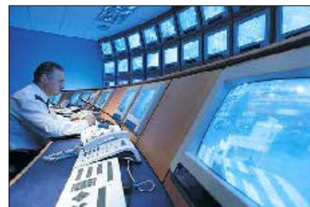
SURVEILLANCE ROOM. MORE THAN 1,000 HIGH-RESOLUTION AND INFRARED CAMERAS MONITORED THE OLYMPICS.
